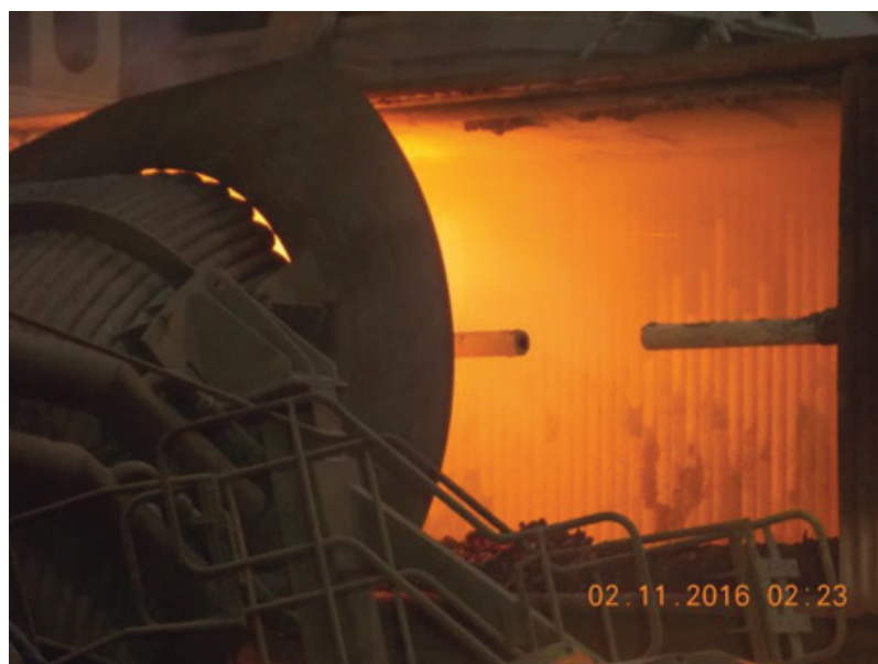
Figure 3. Zolo probes installation at Vallourec Star
